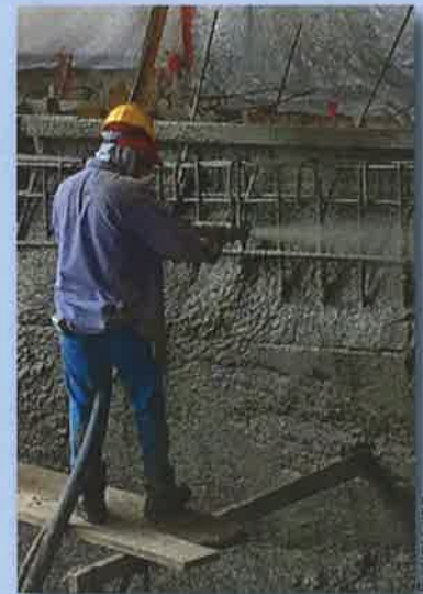
A worker sprays in the side walls of the lap pool in the Margaret Young Natatorium as construction continues towards a spring opening for the indoor, year-round facility.
