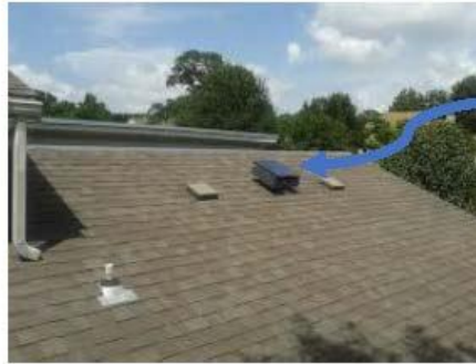
Picture of Solar Vent Fan installed on a roof
