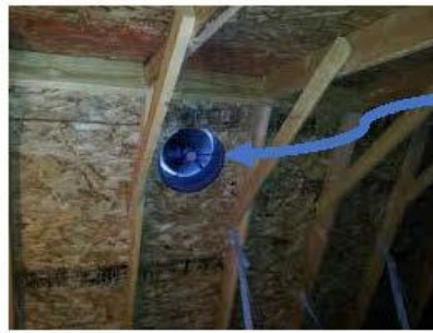
Picture of inside of roof of installed Solar Vent Fan
