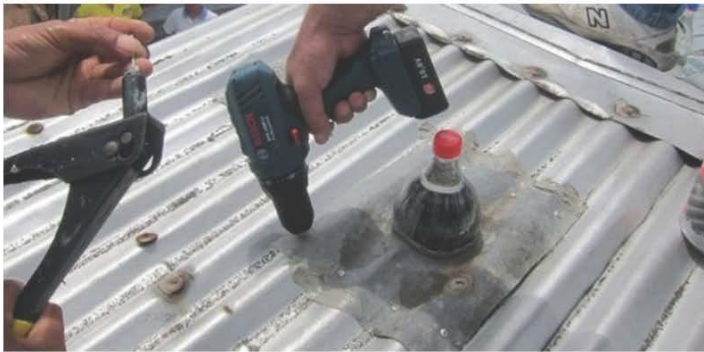
Solar Bottle Bulb – Exterior Roof
