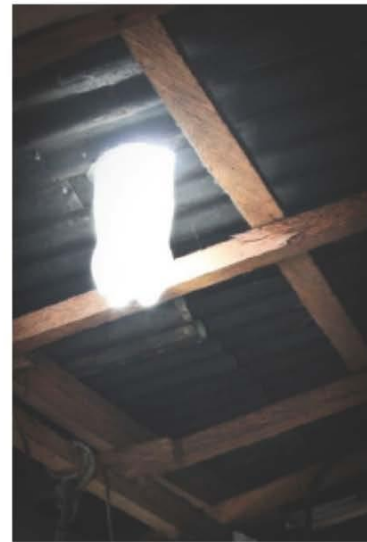
Inside of shed with Solar Bottle Bulb
